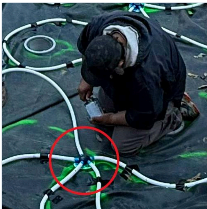
FIG 7.1 Diffuser detail (circled): Sorgiva® diffuser glued to the nozzle at the T-junction of the spider line, with chalked alignment marks on the EPDM.
