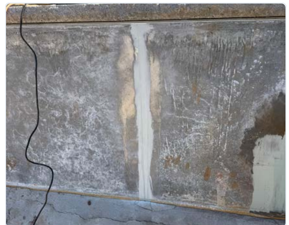
FIG VW.1 Concrete wall after mortar flashing of honeycombing.
